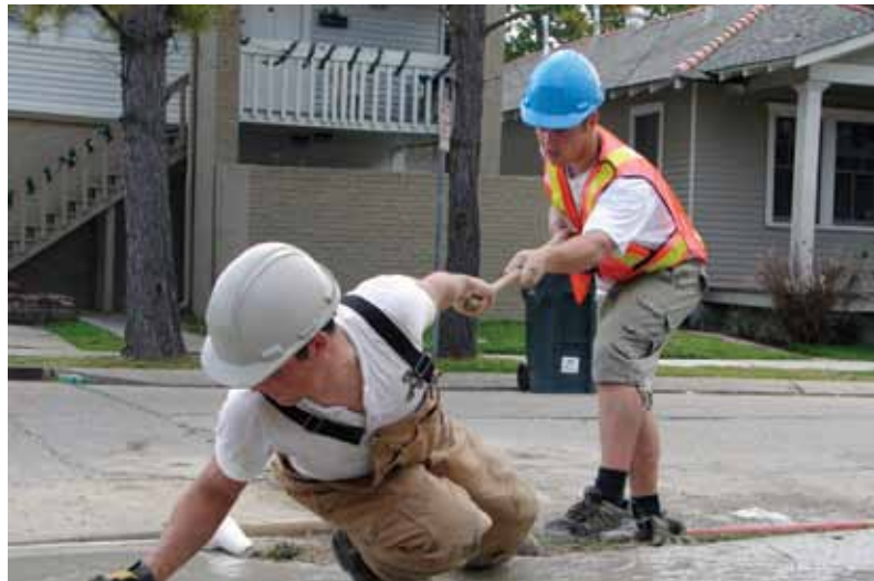
CNA students Ryan Snow and Daniel Roberts show the true meaning of cooperation as they repair a sidewalk in the Broadmoor District.
